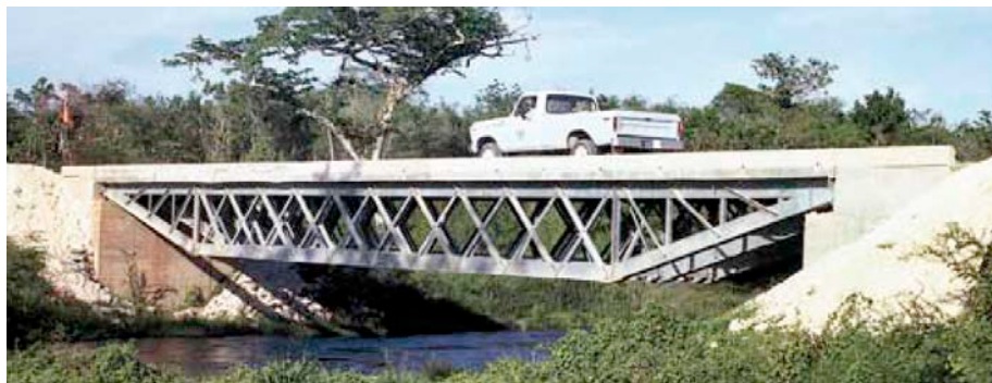
Steel frame truss bridge, located on the Southern Highway, Belize, Central America.
