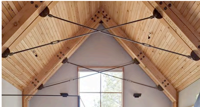
Composite truss roof, Tahoe Ridge House, California. Photograph © WA Design Inc http://www.wadesign.com/newbuilding#/tahoe-ridge-house/
